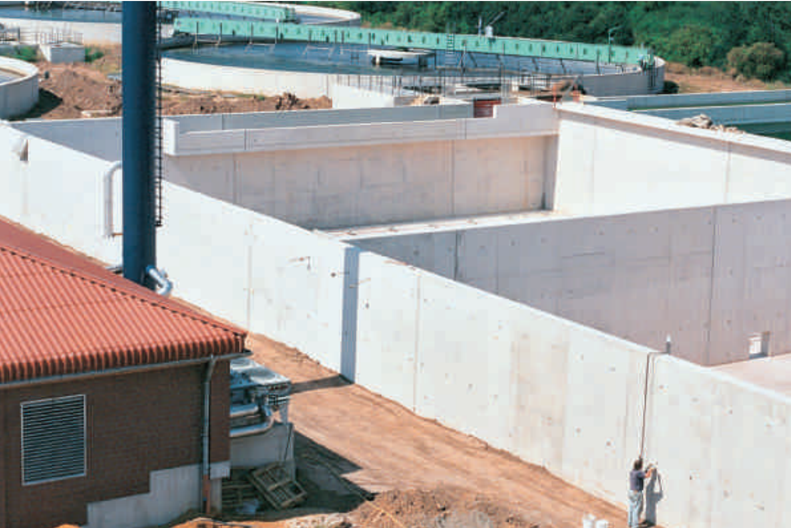
Sewage works in Hameln, Germany.
